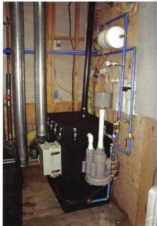
Radon removal system
