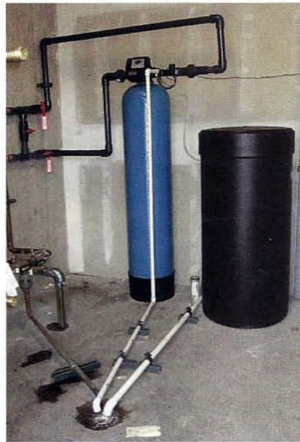
Office building softener
