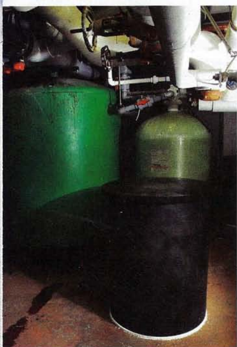
Sheraton® Denver water softener installation
