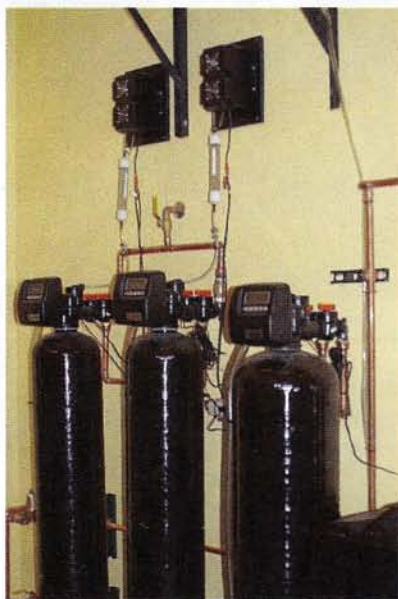
Residential iron removal and softening systems
